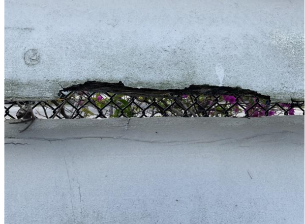
Fence wood rot
