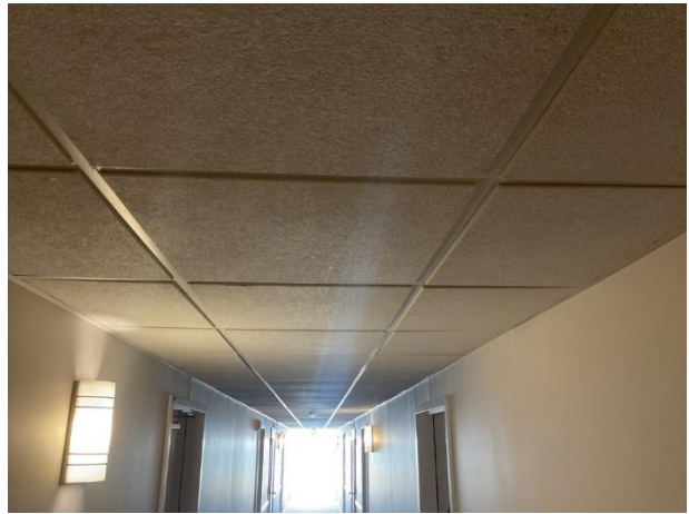
Acoustical ceiling tiles
