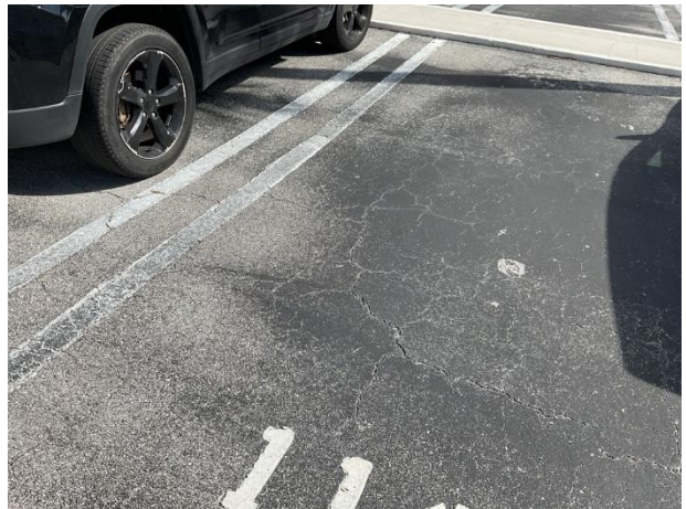
Pavement cracks and seal coat deterioration
