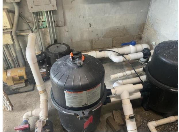
Pool pumps and filters
