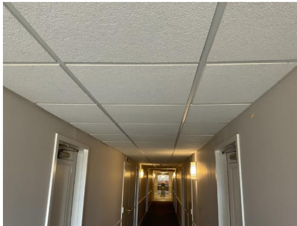
Acoustical ceiling tiles
