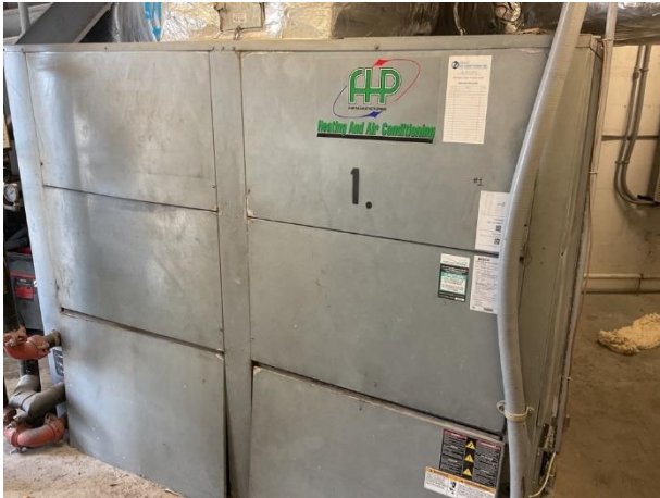
Air handling unit
