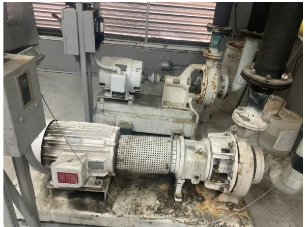
Cooling tower pumps
