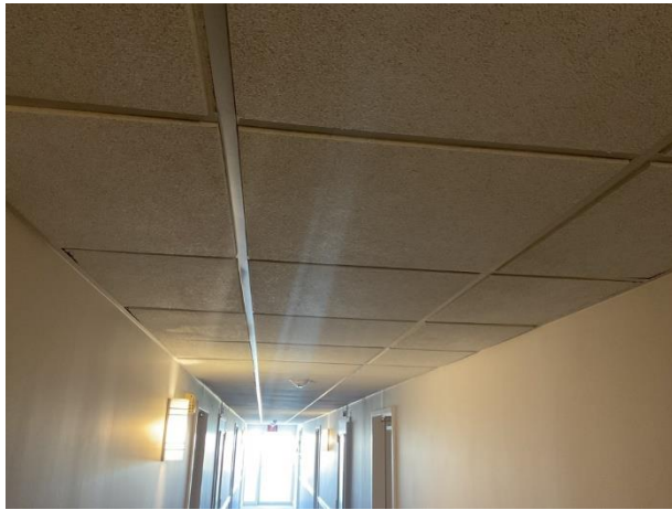
Acoustical ceiling tiles
