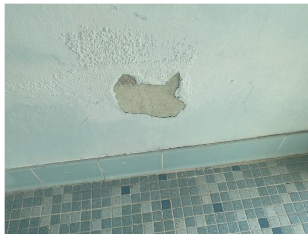
Pool house paint deterioration
