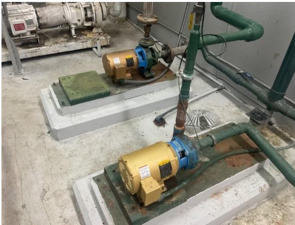
Domestic water pumps
