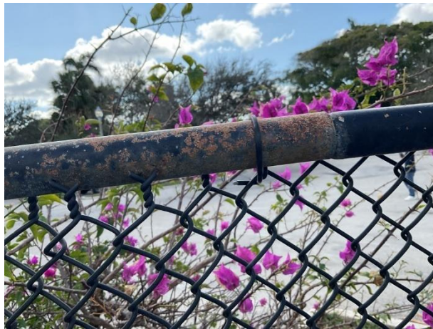
Fence post rust
