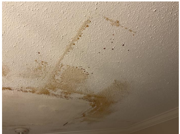
Stains from water damage
