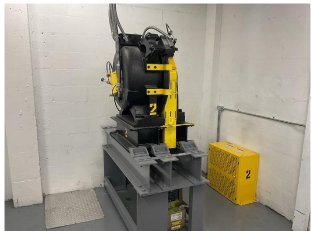
Traction elevator hoist and motor
