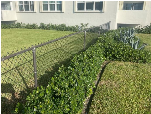
Chain link pool fence
