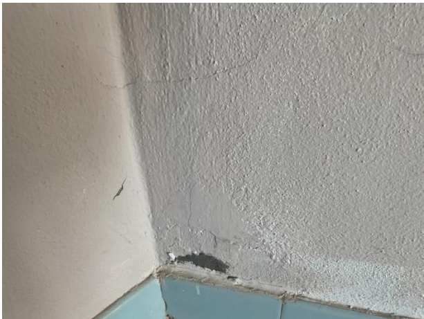
Pool house paint deterioration
