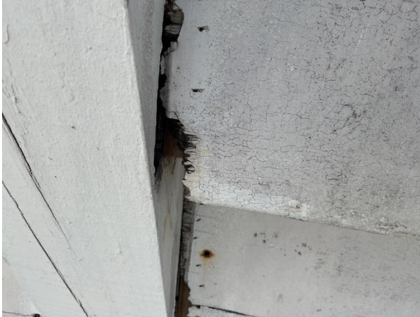
Fence wood rot
