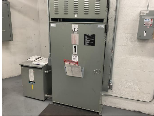
Traction elevator controls
