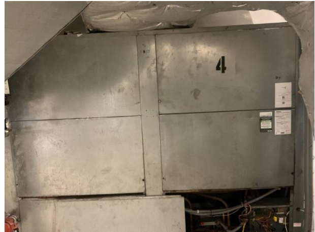
Air handling unit
