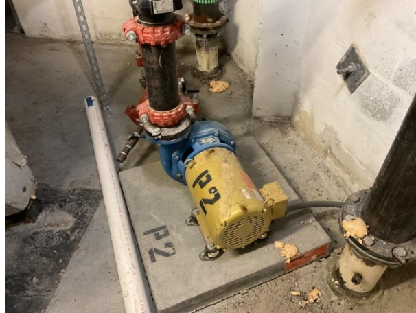
Domestic water pump
