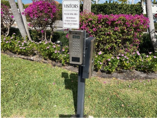
Gate entry keypad
