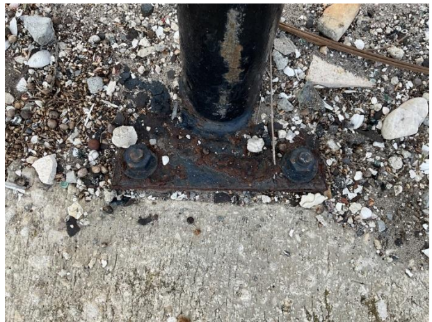
Finish deterioration and rust
