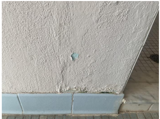
Pool house paint deterioration
