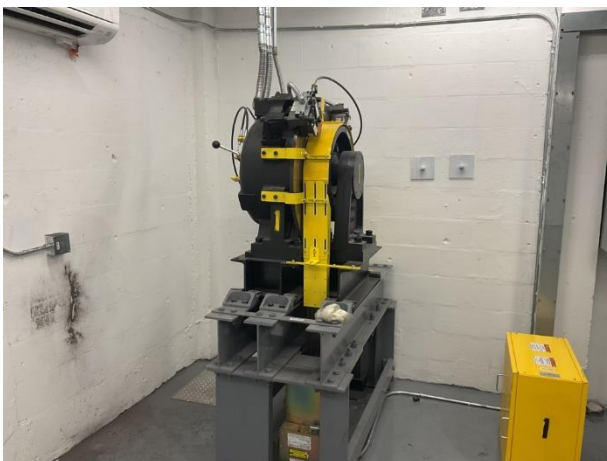
Traction elevator hoist and motor
