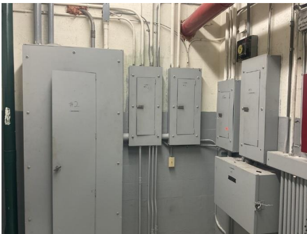
Electrical system main panels
