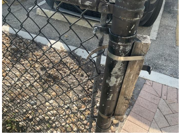
Fence coating deterioration
