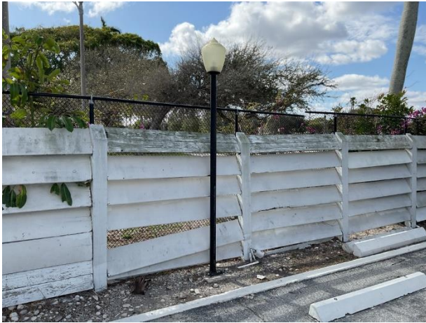
Light pole and fixture
