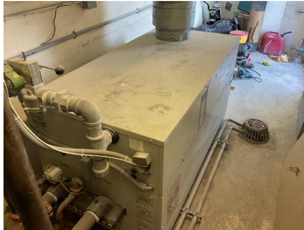
Building heat boiler
