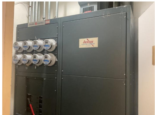
Electrical system components
